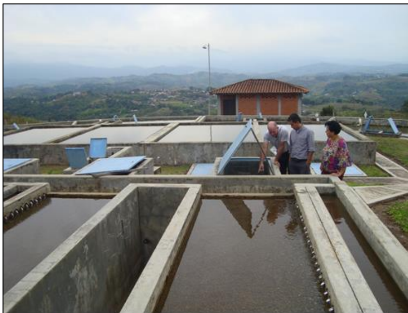
Figure 2. The community-managed water treatment plant in Mondomo. Source: DESAFIO's team in UNIVALLE, Colombia.
